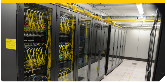
Top Super Computer racks in the control building of the Murchison Radio-astronomy Observatory (MRO). Credit CSIRO.
